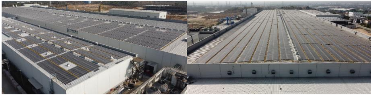
6.61 MW solar rooftop plant
