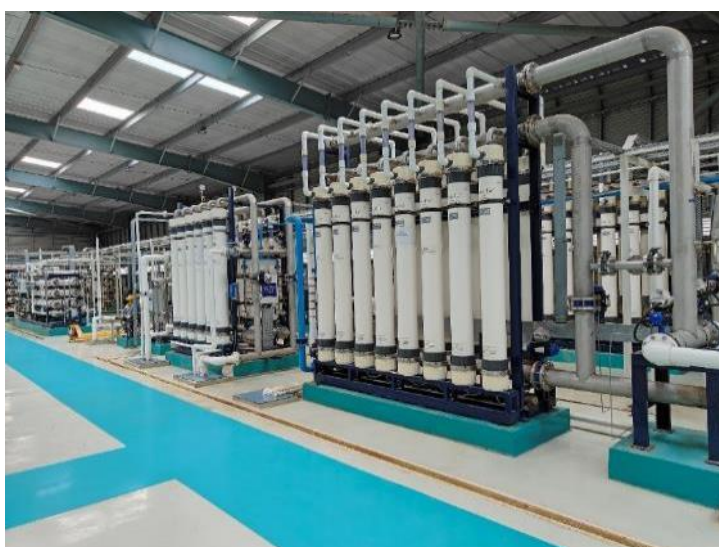
Ultra-pure water generation plant at Unit II
